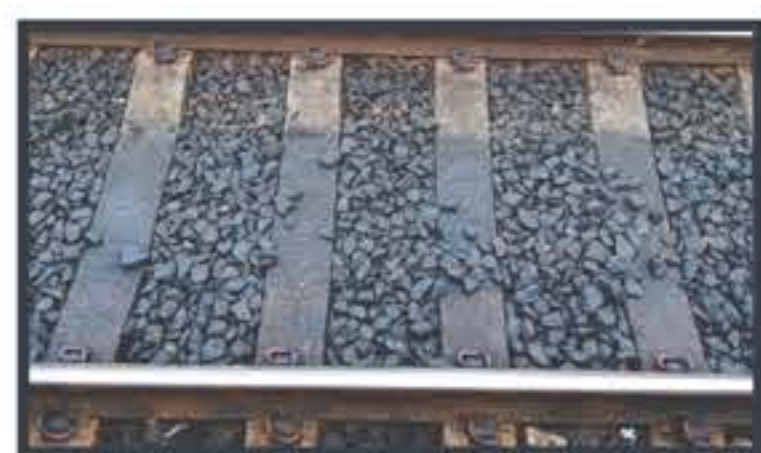
Fig. 1: example of diesel contaminated railway ballast
